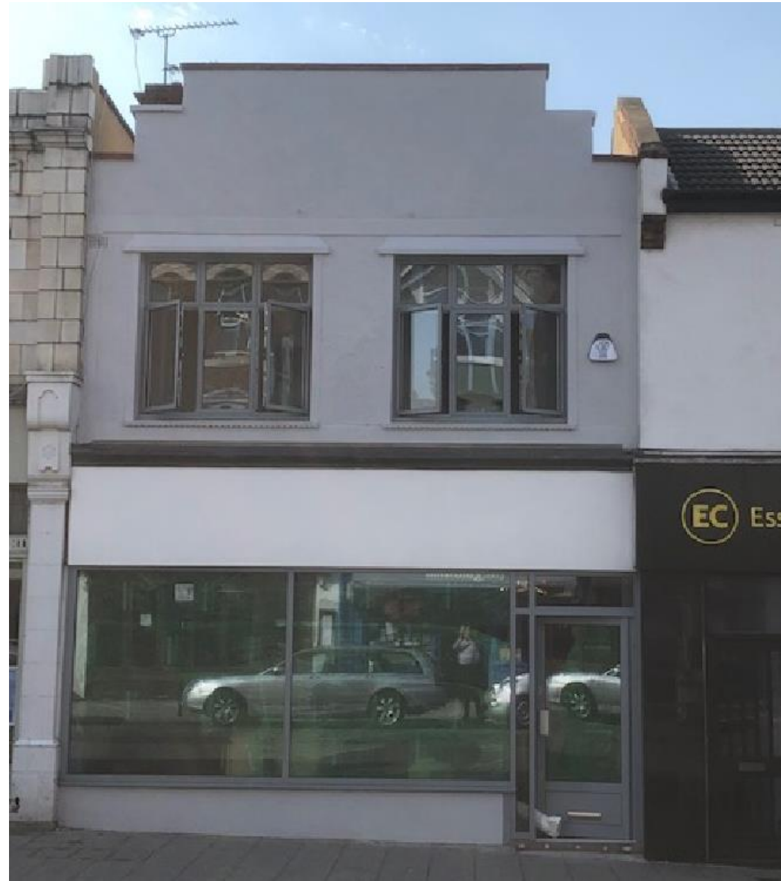
Unauthorised Change to aluminium and UPVC in 2019 – newly completed
